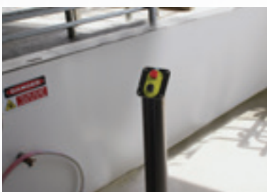
Platform Operator Console - E-Stop Can be activated in case of an emergency
