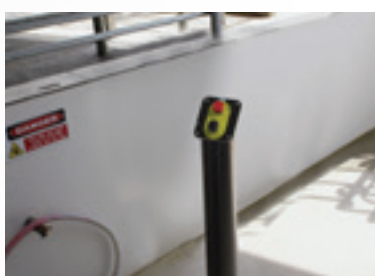
Platform Operator Console - E-Stop Can be activated in case of an emergency
